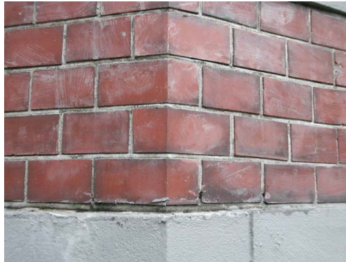
Fig. 1: Red brick-like tile used for the façade of the Governor General Building, Taipei, Taiwan.
